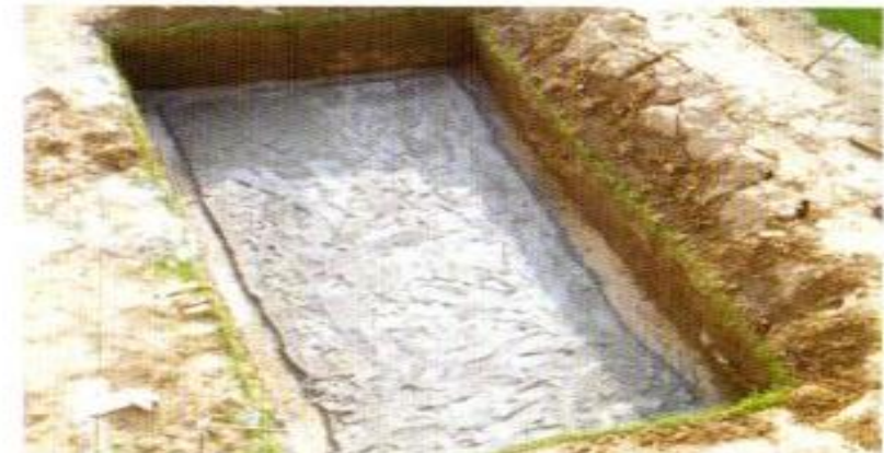
3. Preparation of Ground after excavation with PCC/RCC on the floor before placing the swimming pool.
